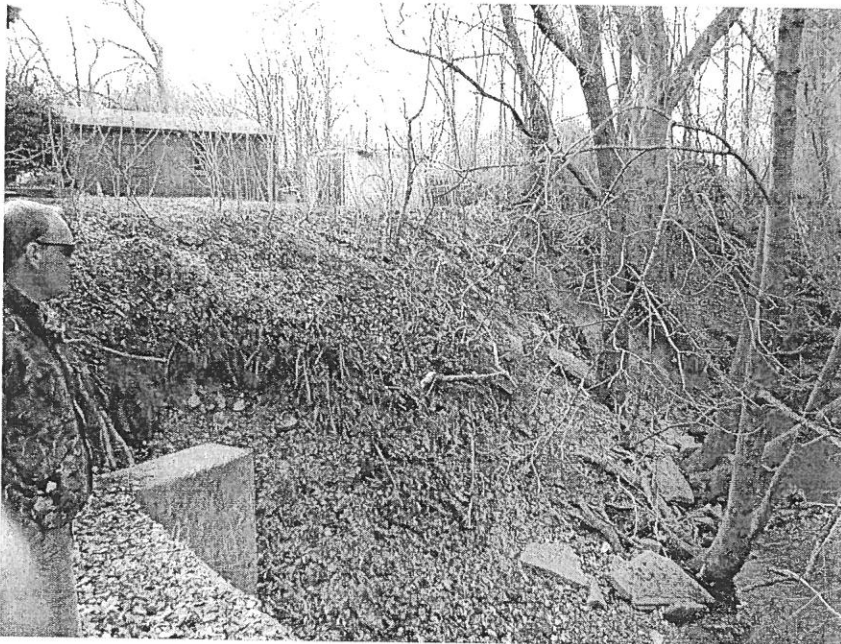
1 Erosion at Indian Steps, Possible Mitigation Project
